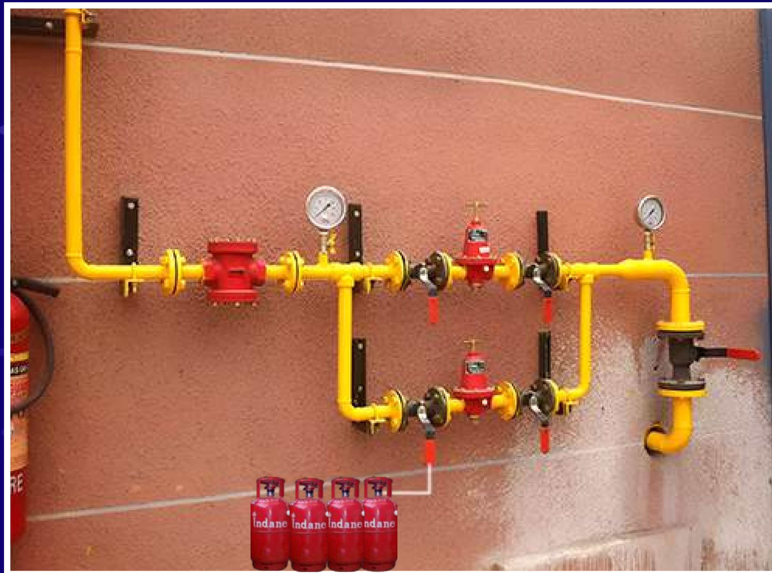
GAS CYLINDERS PIPES
